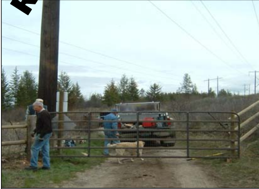
Michael Haywood, Dale Truitt and Jake Van Holland replacing the power line gate near Harvard Rd. (gate had been vandalized)
